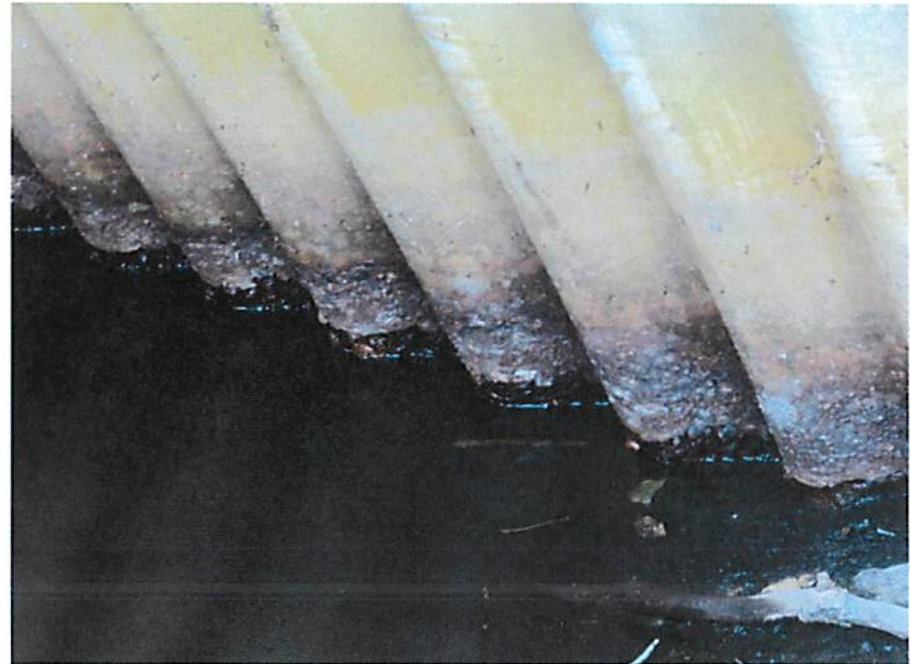
Typical rust Notes
