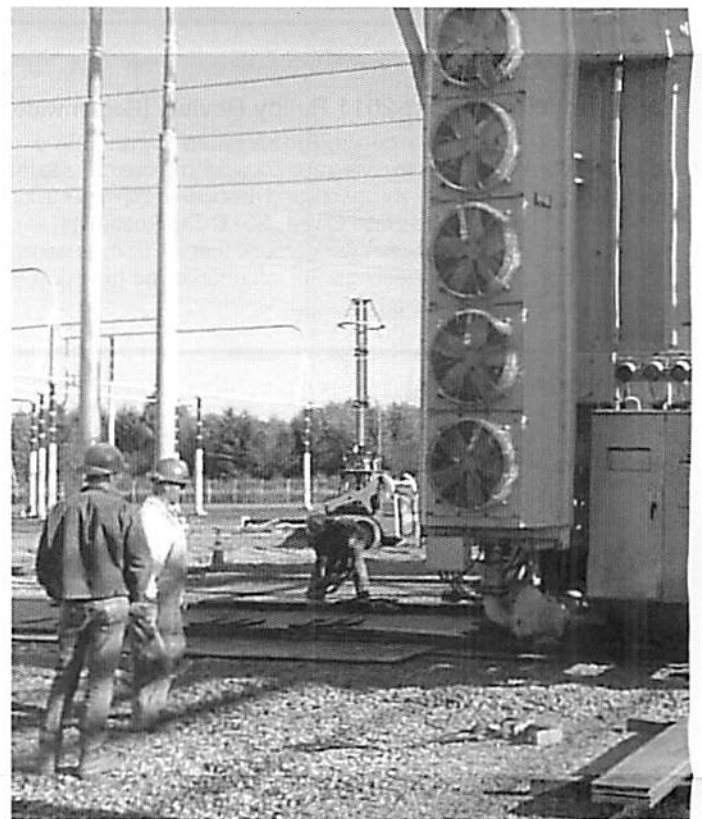
BPA's rigging team moves a massive transformer at Custer Substation. To read more or watch a video, go to bpa.gov/news/newsroom/Pages/How-does-BPA-move-a-transformer-Verrrrrry-carefully.aspx
