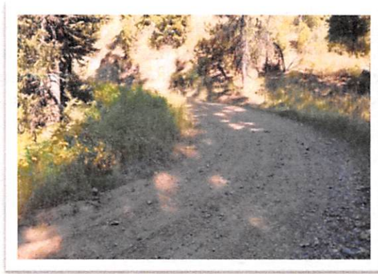
Photo 5: Road in Nez Perce Fork – Nelson Lake watershed with areas of surface erosion.
